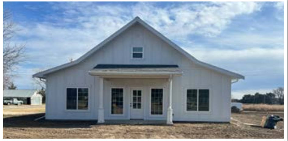
The new housing project in Alton is nearing completion with work underway inside by Nation Builders Ministries.
